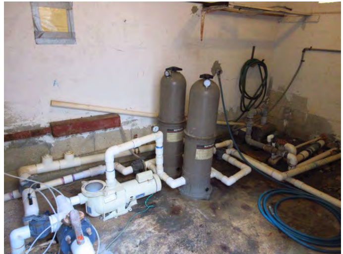
GENERAL VIEW OF SWIMMING POOL EQUIPMENT
