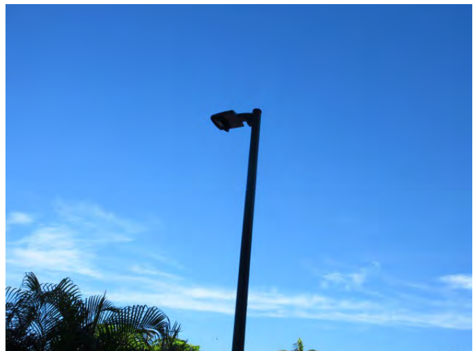
VIEW OF SITE LIGHTING
